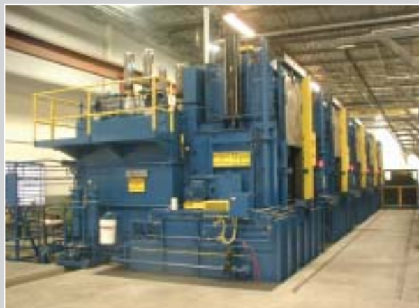
Turnkey complete UBQ system installation and integration.
